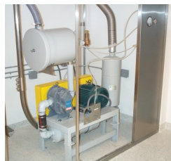
Central Vacuum Pump Unit
